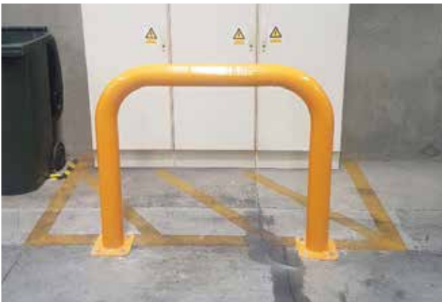
Steel Hoop Bollard protecting critical factory plant from damage.
